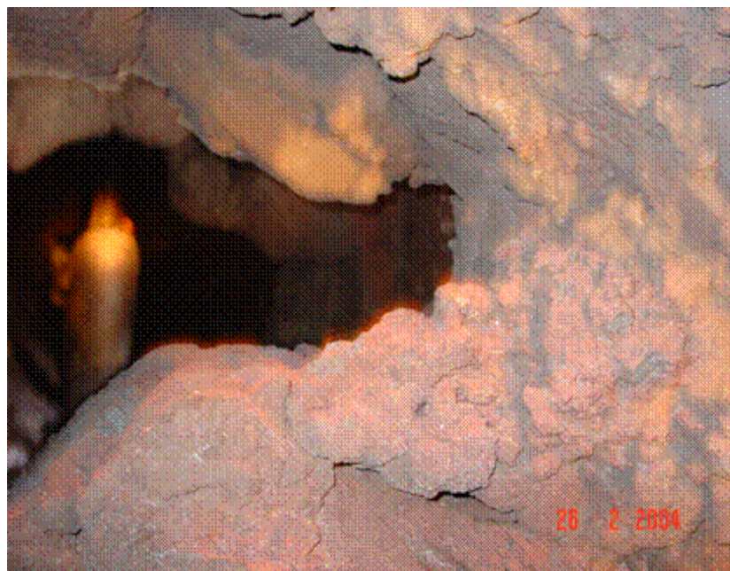
Figure 25.3: Extensive accretion formation in rotary kiln
