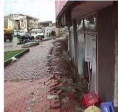
Damaged pavement, Chi-Chi
