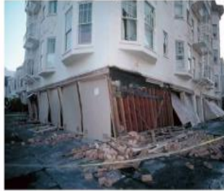
Soft first story/inadequate shear strength
