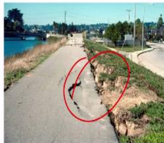
Ground failure due to liquefaction, Loma Prieta earthquake. (Photo from: http://earthquake.usgs.gov/bytopic/photos.html )
