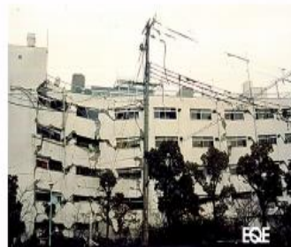
Kobe earthquake damage. Failure of the first story caused partial collapse of upper stories. ( http://www.eqe.com/publications/kobe/kobe.htm )
