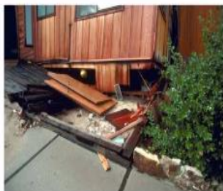
Column failure, Loma Prieta earthquake. (Photo from: http://earthquake.usgs.gov/bytopic/photos.html )
