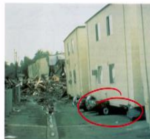
Heavily damaged apartment building, Northridge . The building has collapsed onto its structurally weak first story, partially crushing several parked cars. This type of damage was common in the epicentral region; partially open first-story levels have poor resistance to strong, horizontal ground motion. The piles of debris and the destruction on the left are the results of a fire that broke out after an aftershock. Photograph by J. W. Dewey.
