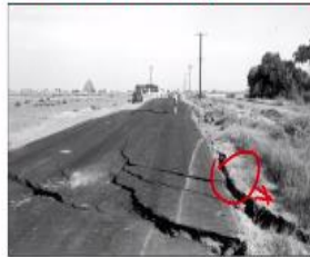
Lateral spread at site 13 on Heber Road (location shown on Plate 1, Professional paper 1254), showing associated displacements, fissures, and sand boils. The pavement on Heber Road settled, cracked, and shifted to the south by as much as 1.2 meters. View is east.
