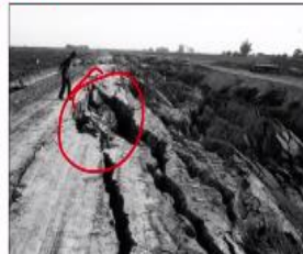
Slumped banks of the Barbara Worth Drain at site 30 (location shown on Plate 1, Professional paper 1254). The slump in the east bank destroyed a farm lane and blocked the drain. View is south.
