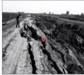
Slumped banks of the Barbara Worth Drain at site 30 (location shown on Plate 1, Professional paper 1254). The slump in the east bank destroyed a farm lane and blocked the drain. View is south.
