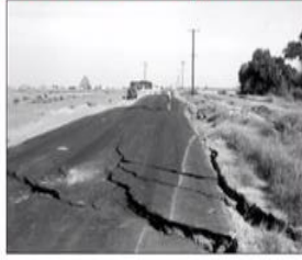
Lateral spread at site 13 on Heber Road (location shown on Plate 1, Professional paper 1254), showing associated displacements, fissures, and sand boils. The pavement on Heber Road settled, cracked, and shifted to the south by as much as 1.2 meters. View is east.
