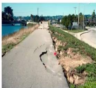
Ground failure due to liquefaction, Loma Prieta earthquake. (Photo from: http://earthquake.usgs.gov/bytopic/photos.html )
