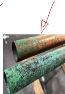
Corroding copper pipes
